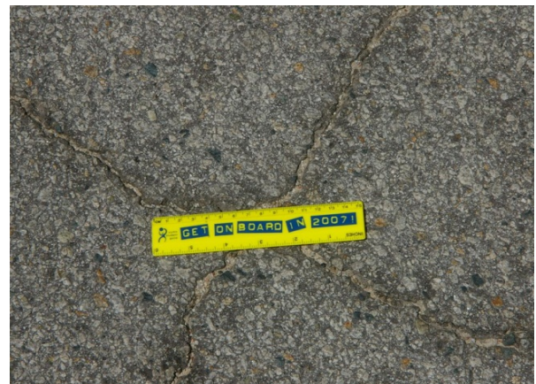
Fig. 3. Moderate severity block cracking.
